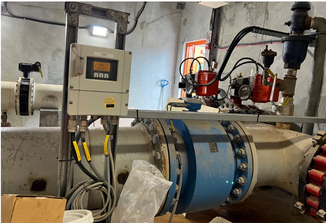
La station de pompage.
